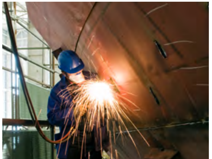
Welding new steel plates on a ship's hull during repair work on a ship in a dry dock.
